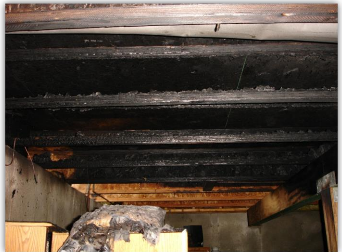
Complete burn thru of OSB web. 1 st flooring decking being supported only by the chords.
