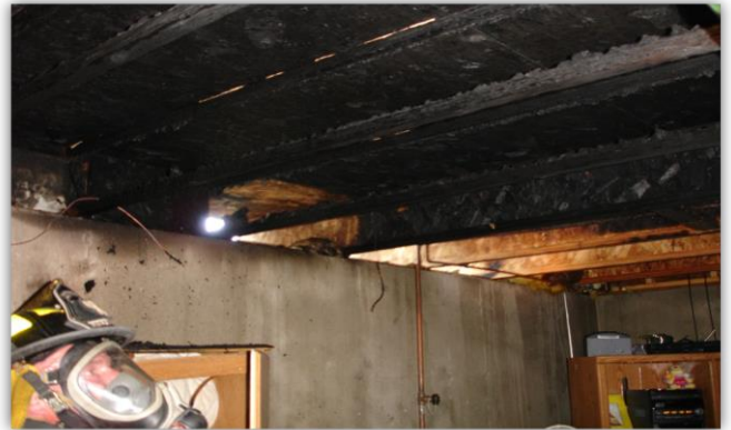
Basement view showing unprotected TGIs.
