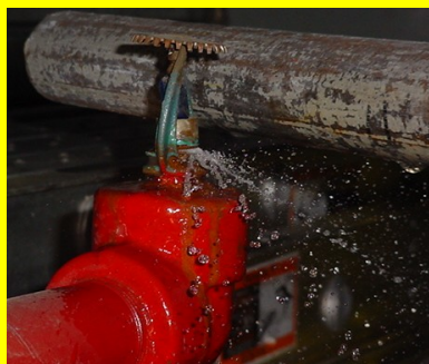
DAMAGED FRANGIBLE BULB HEAD
