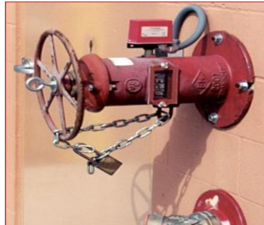
WALL POST INDICATOR VALVE w/ TAMPER SWITCH * note OPEN
