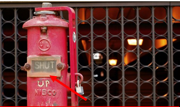
SHUT and secured with padlock.
